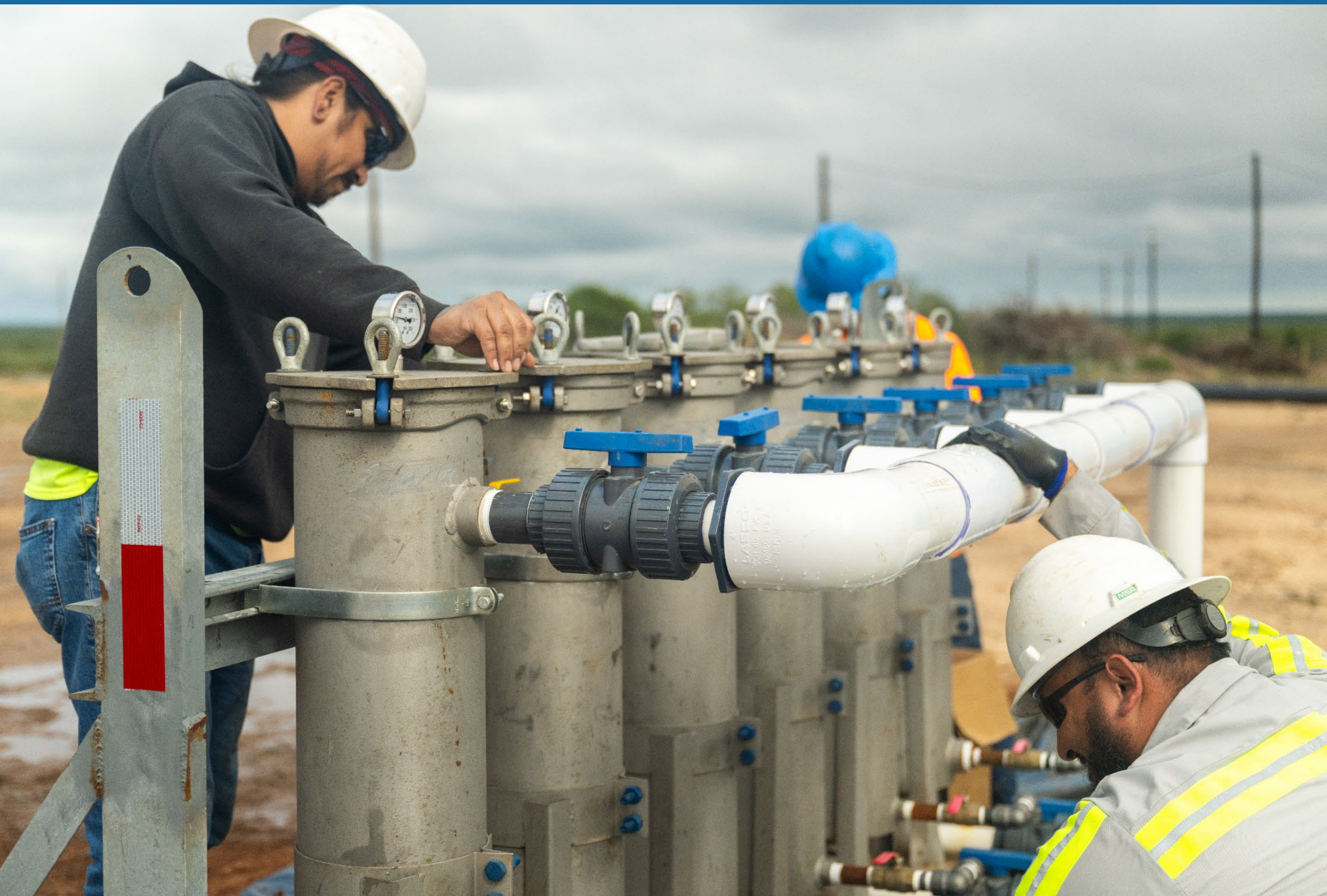
Rosita ISR Uranium Central Processing Plant
