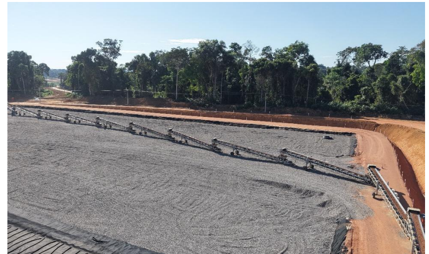
Mobile conveyors transporting agglomerated ore from the agglomerating drum to pad 1
